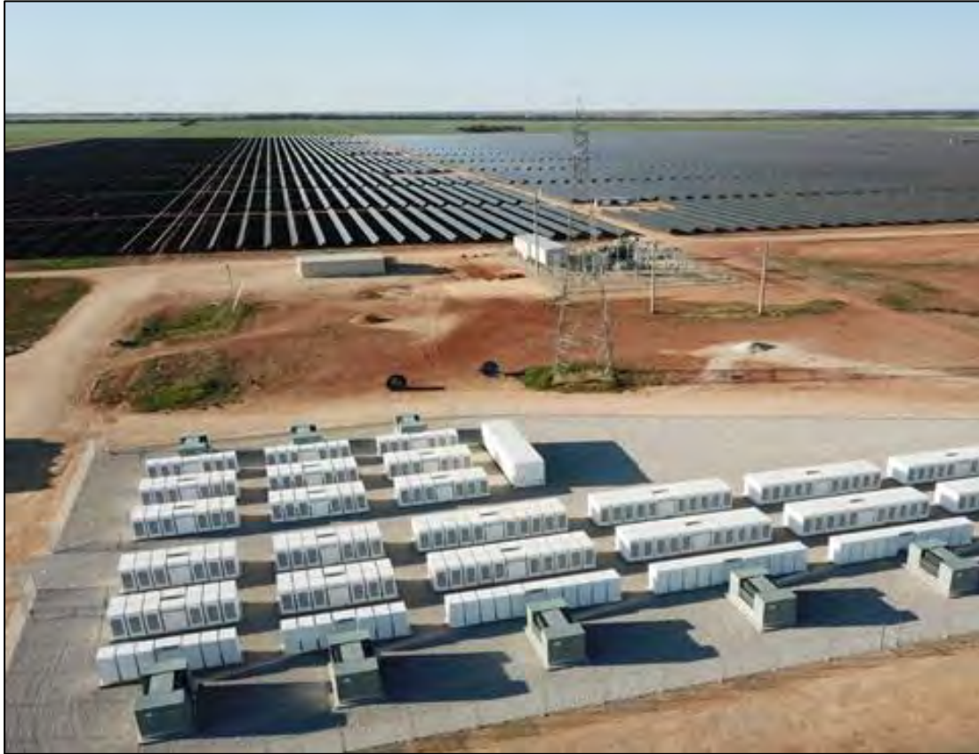
Figure 13 - Indicative battery storage system enclosures (Edify's Gannawarra Solar and Battery project)
