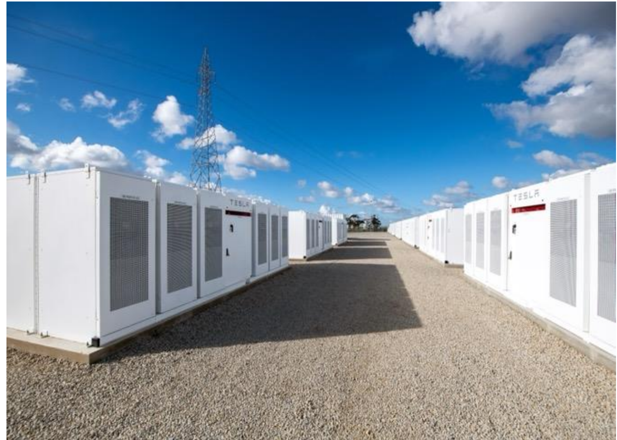
Edify's Gannawarra Energy Storage System
