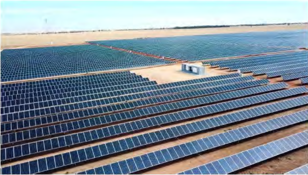
Figure 2-10 Solar arrays and inverter (example). A distributed BESS system would include battery installations alongside inverters (Source: Edify Energy, 2020)
