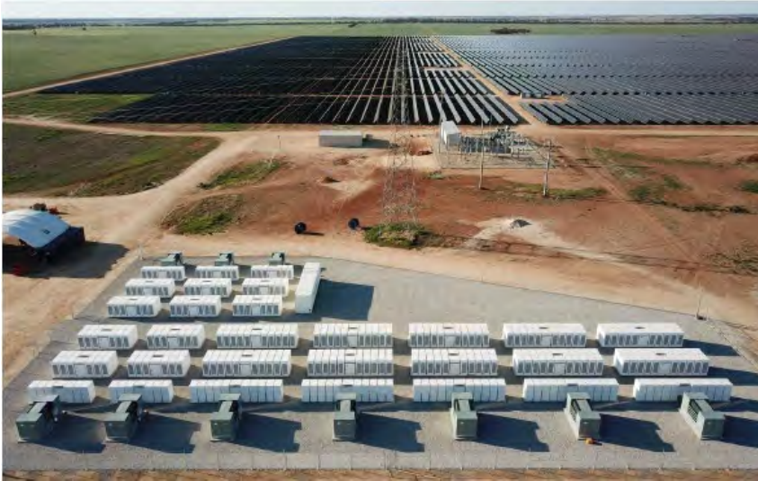
Figure 2-8 Consolidated battery installation example (Source: Edify Energy, 2020)
