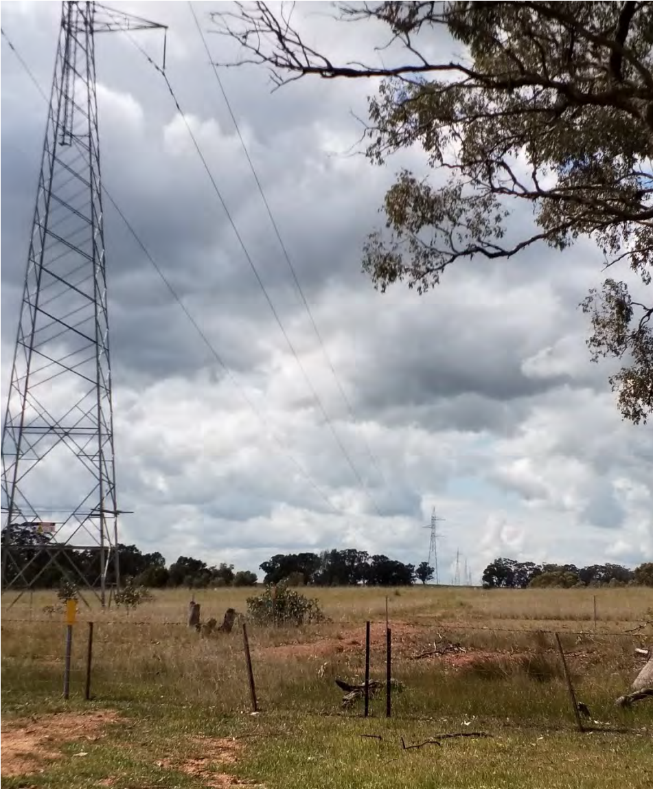
Figure 2-14 Existing 220kV transmission lines (and underground cable) traversing the proposal site
