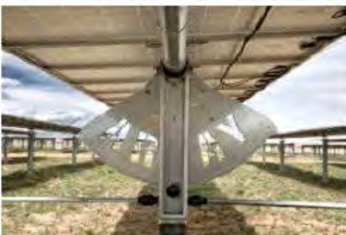
Figure 2-4 Solar array example (Source: Edify Energy, 2020)
