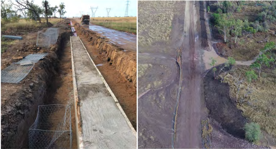
Figure 13. Example of a low profile causeway across a watercourse on previous Edify projects (left) under construction and (right) following rainfall.
